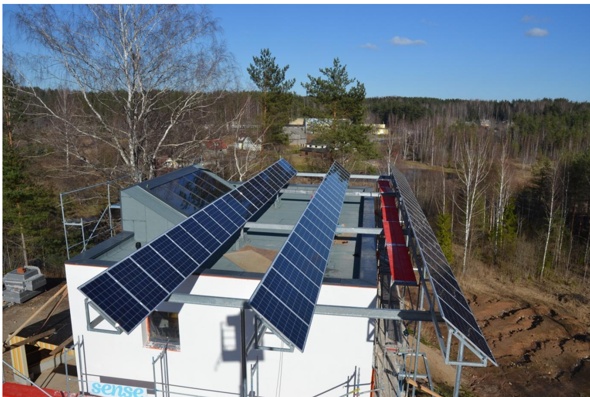
Figure 4 Roof with mounted PVs. Solar thermal collectors on the left.
